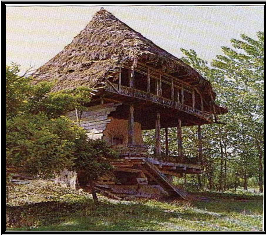
Figure 6. A village house based on wood, affected by landslide.
